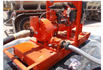
High Head Pumps for Temp Fire and Cleaning
